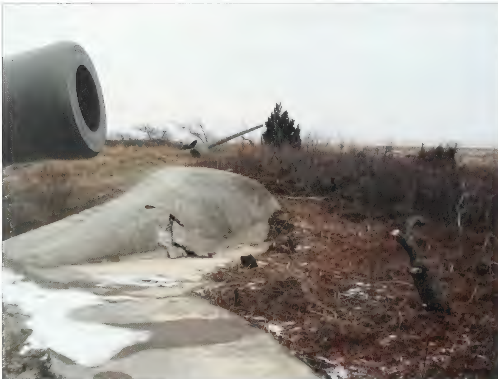
Figure 3.43. View looking north from emplacement #1 to emplacement #2, Battery Gunnison. Spalling is present on a concrete feature due to infiltration of water and freeze-thaw cycles (Olmsted Center, January 2009).
